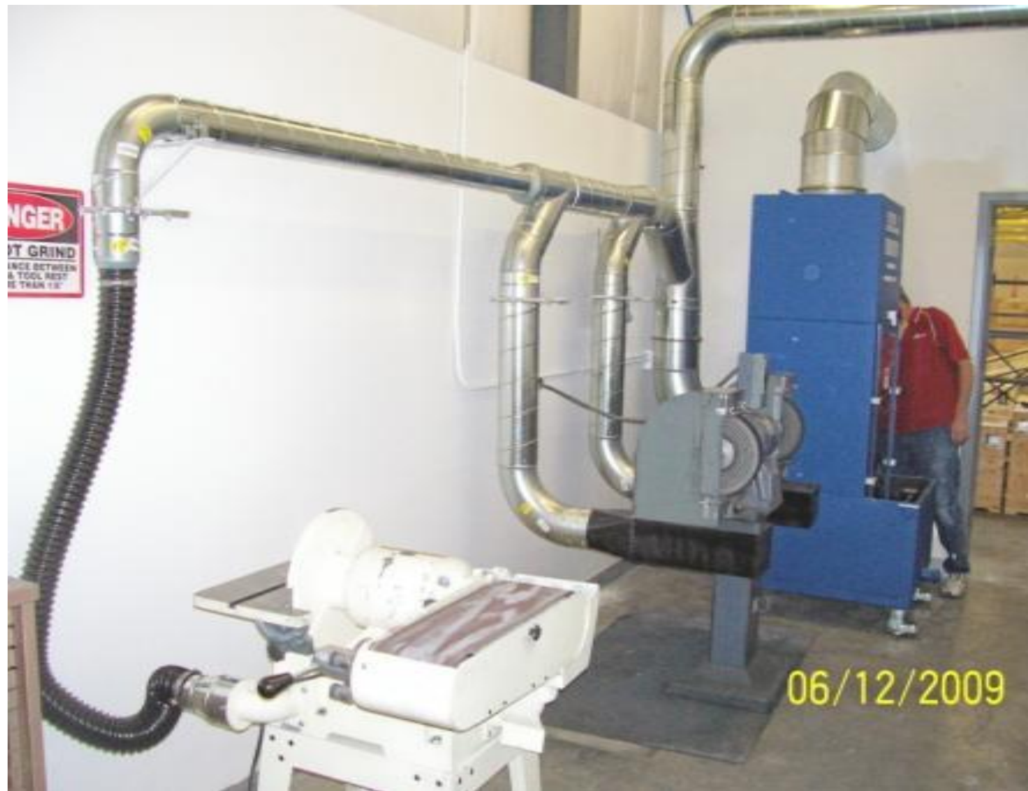
Wet Ducted Collector
