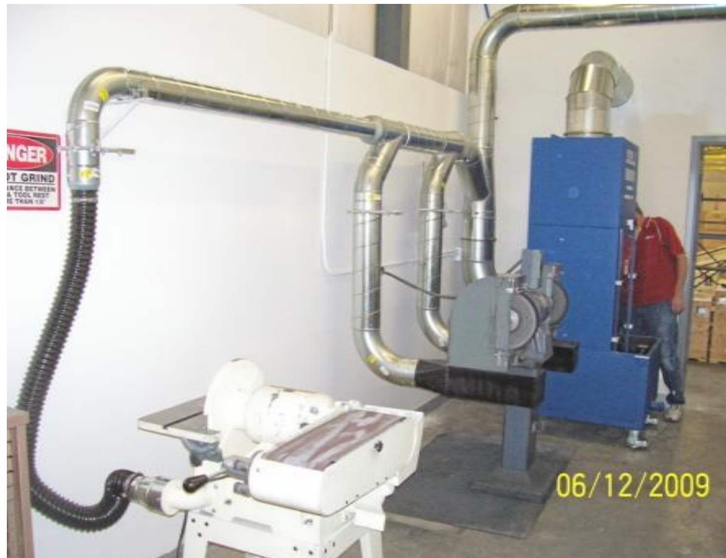
Wet Ducted Collector
